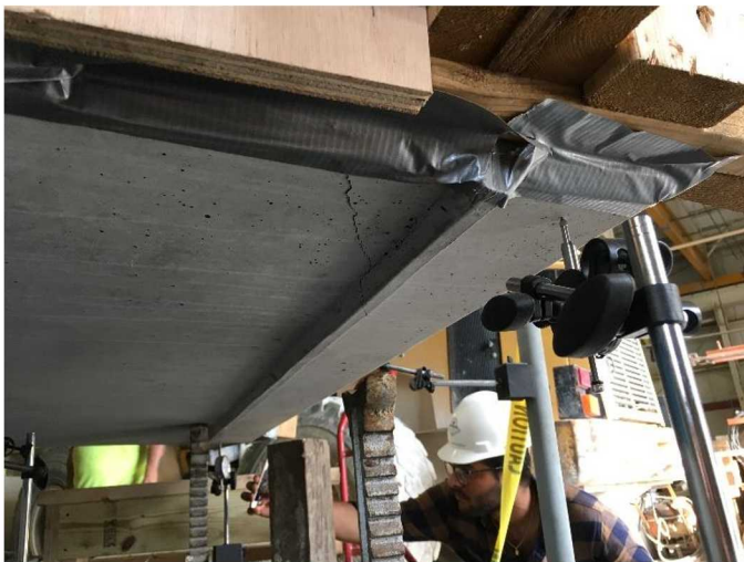
Figure 5: Side view of crack after deck pour and accidental overload
