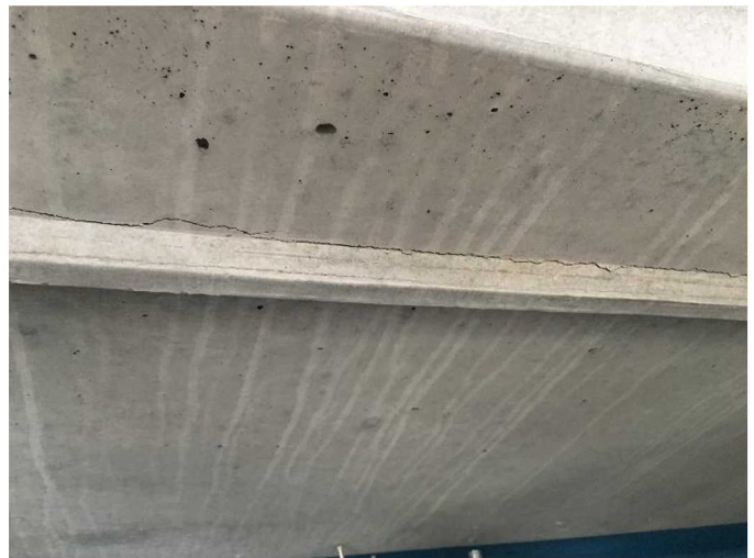
Figure 6: Front view of crack after deck pour and accidental overload
